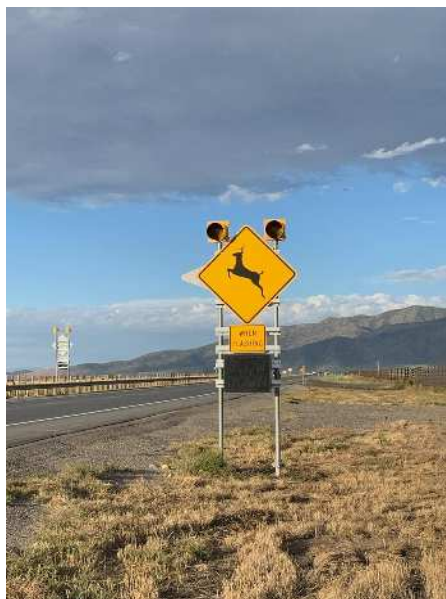
写真 2-2-33 LED 警告標識
